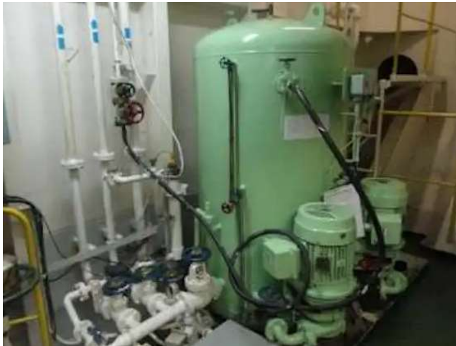
Gambar 1. Sistem pompa air tawar [6]
